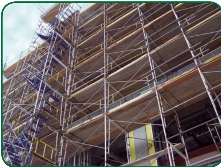
Exposed wood scaffold planking is a considerable investment on any job site.
